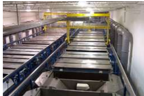
Figure 3: Automatic lines with covered tanks incorporated with the exhaust system.
