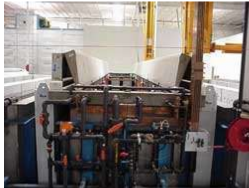
Figure 1: Tank with cover open.
